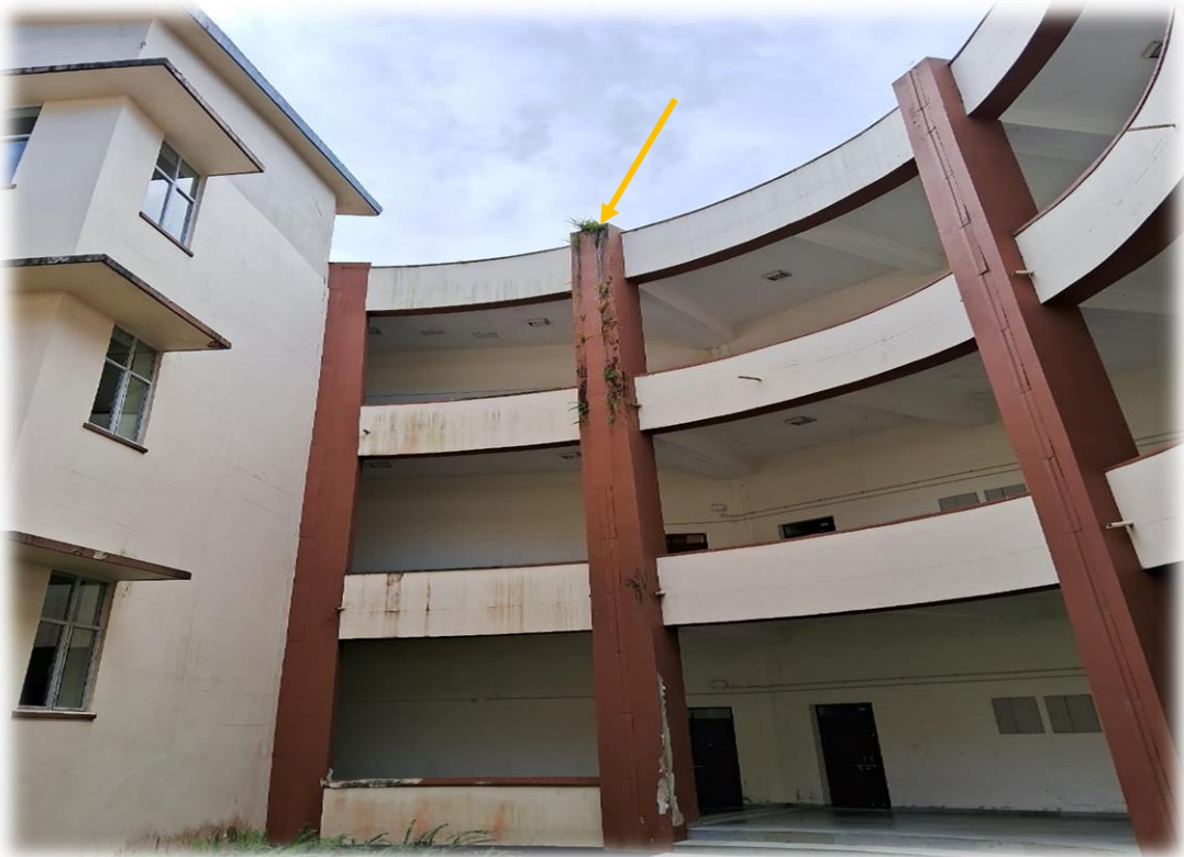
Plants are starting to grow in between the cracks.
